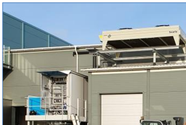
Condensing unit for BUUS 24 ton / 24h flake ice plant. CO2 DX.
